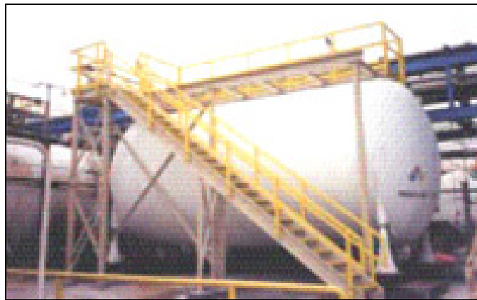
Figure M11.36: Fiberglass ladder system
