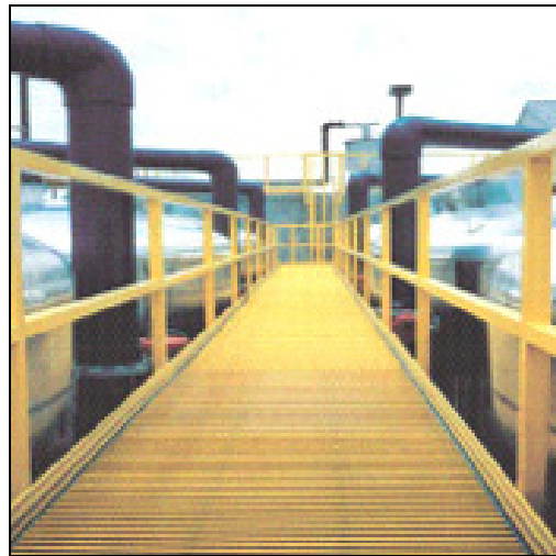
Figure M11.34: Composite handrails and grids/gratings
